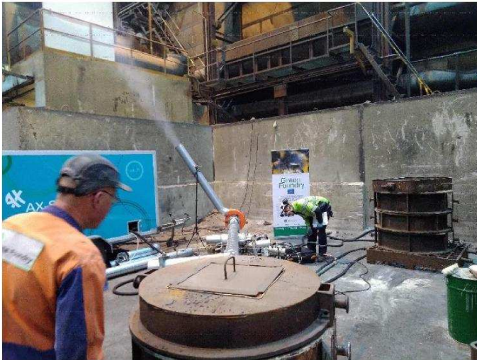
Photo 36. Chamber test after closing the cover.
