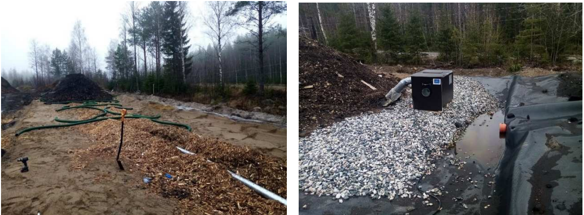
Figure 22-23. Left: Aerating and heating system pipelines in the base of the composting test heaps. Right: Fan for heating and aerating and a dam for collecting wastewater samples.
