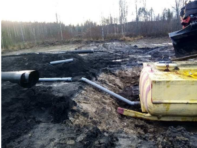
Fig. 6 Waste water collection pipelines and a container.
