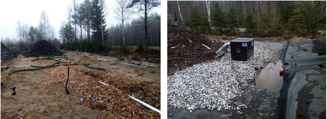
Figure 22-23. Left: Aerating and heating system pipelines in the base of the composting test heaps. Right: Fan for heating and aerating and a dam for collecting wastewater samples.
