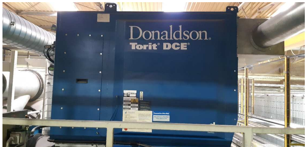
Picture 3. Donaldson fiber filter installed in the exhaust air of the discharge site
